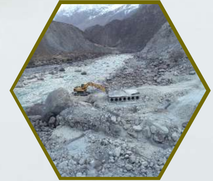
Hanzel Hydro Power Project Gilgit Baltistan
