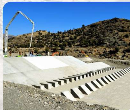
Dhana Irrigation & Water Supply Scheme
